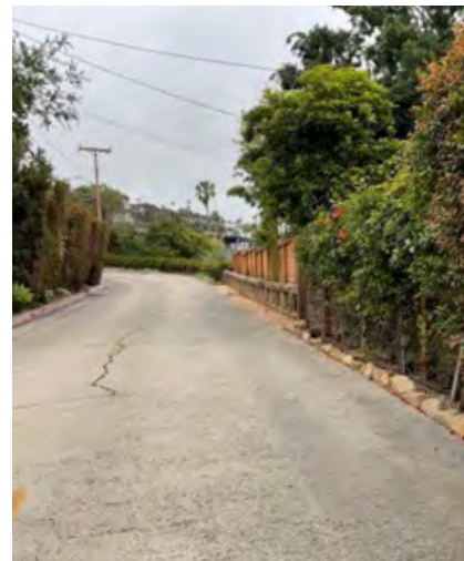
After fence and ivy have been removed from Pier and Cap Wall
