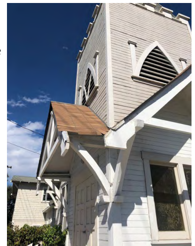
Newly named historic landmark, St. Paul's AME Church in need of repairs. Photo by Steve Dowty
