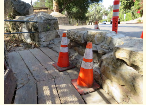
Initial inappropriate repair, June 2022
