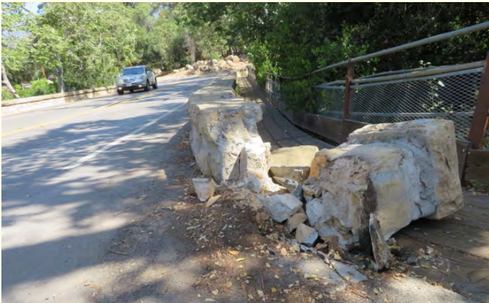
Damage due to automobile accident, May 2022
