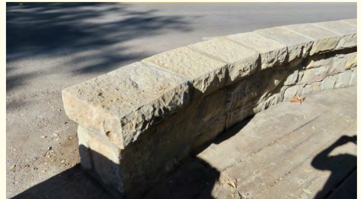
Professional repair that reflects the skill of the master stonemason, whose sensitivity reflects the historic style of the stonework, the historic color of the sandstone and mortar, as well as the historic width of the mortar, November 2022.
